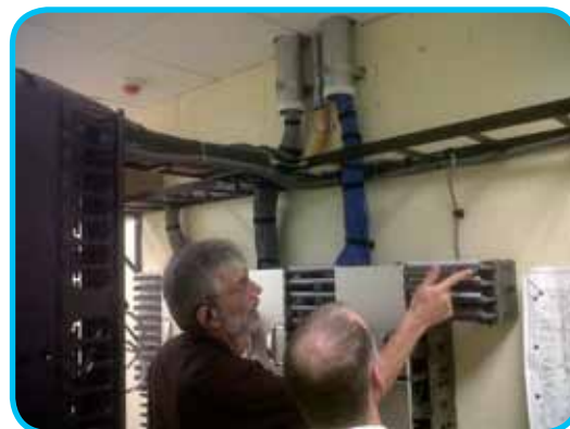
AFL completes work in one of four IDF rooms by testing data and fiber cables that will connect workstations to the Wells Fargo network.
