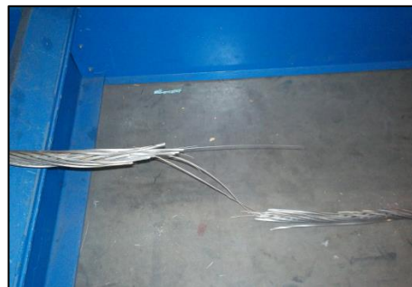
Conductor break at Mid-Span
