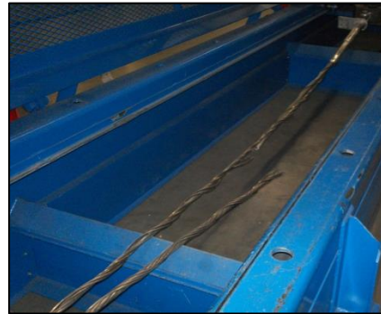
Conductor break at Mid-Span
